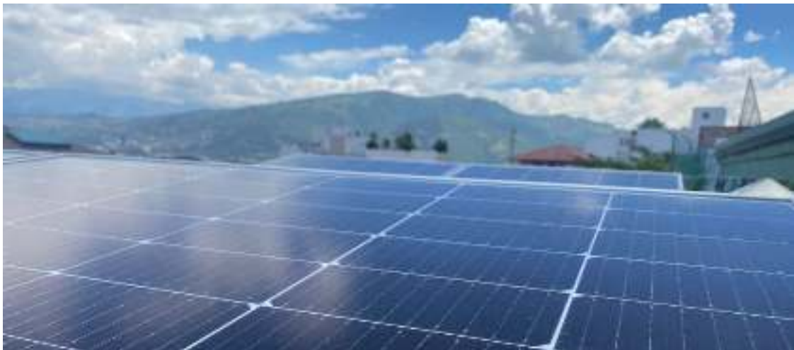
Figure 1. Solar Panels at campus
